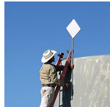
Wireless antenna and camera installation
